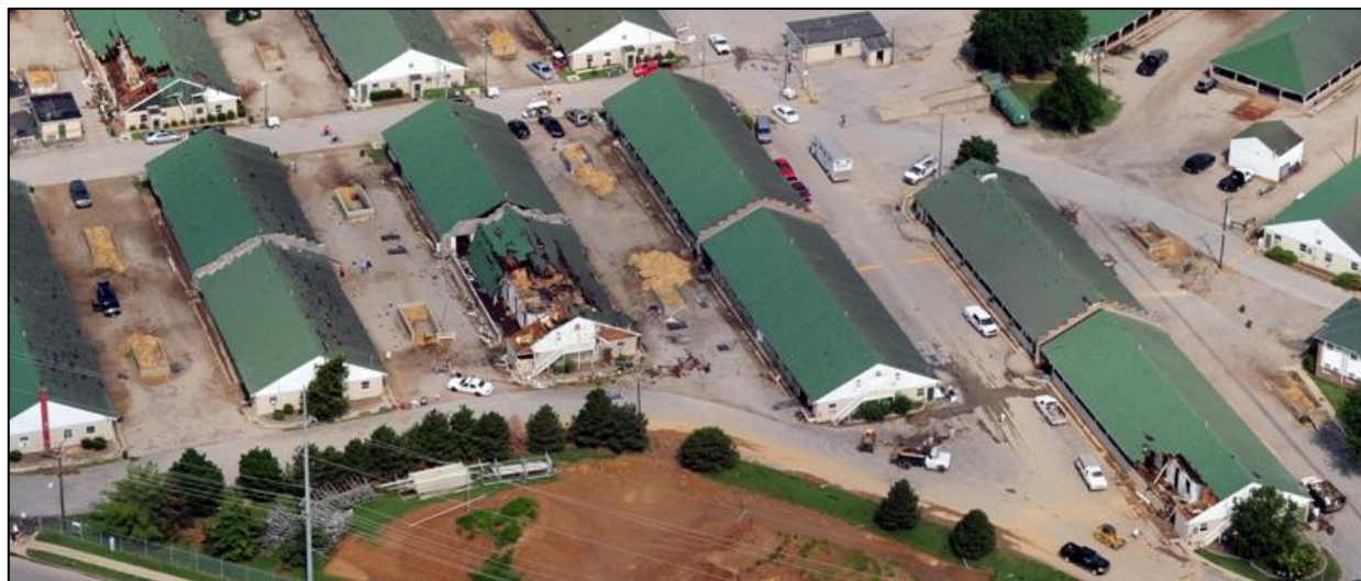
Damage to horse barns at Churchill Downs.
