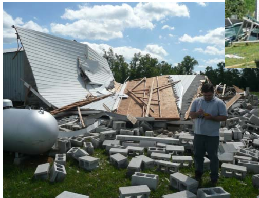
Left: NWS storm surveyor records information about tornado damage in Edmonson County. NWS
