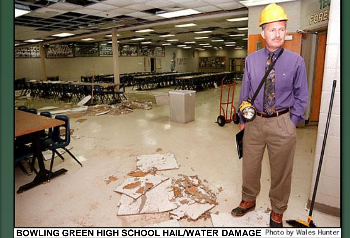
BOWLING GREEN HIGH SCHOOL HAIL/WATER DAMAGE Photo by Wales Hunter
