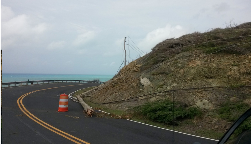
Fig. 19. Broken light pole at Turners Hole and Grass Point on Route #60, St. Croix.
