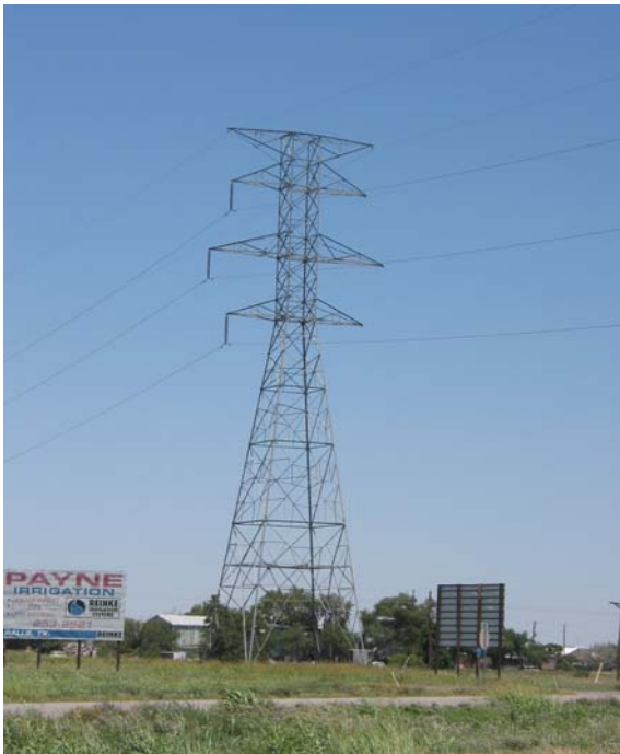
ETL: Metal Truss Tower
