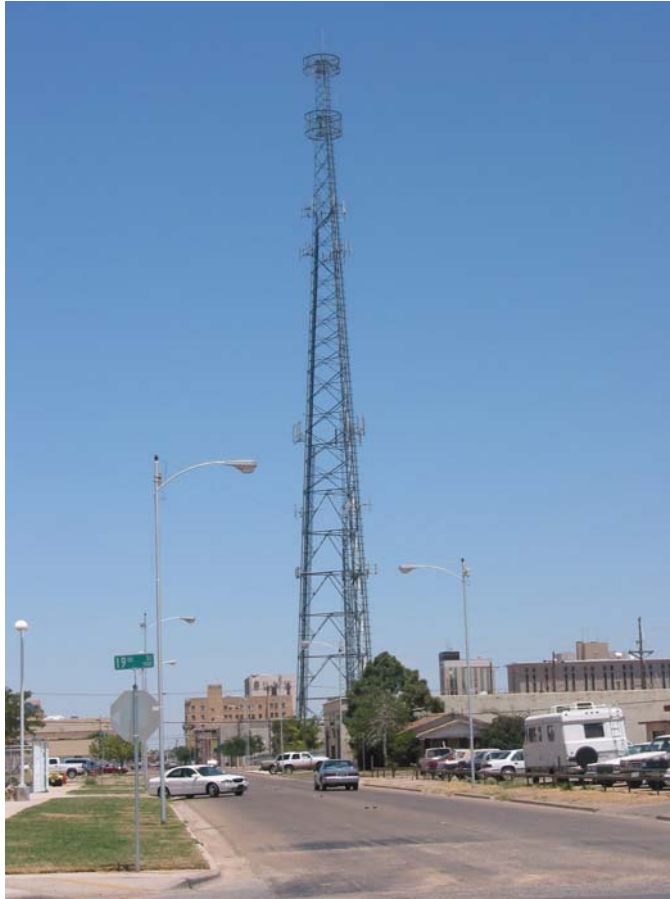
FST: Free-standing Truss Tower
