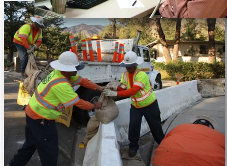
Los Angeles County Public Works deploying K-Rails below burn area prior to expected heavy rains (Photo credit: Getty Images)
