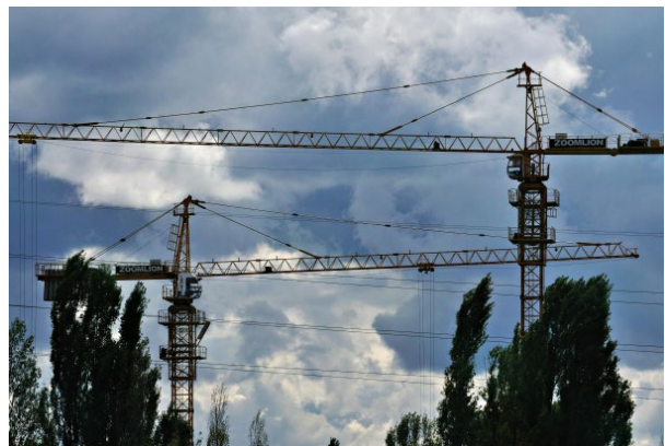
Figure 3: Cranes are especially vulnerable to lightning.
