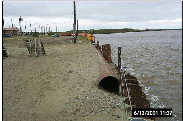
Obvious outward bowing of wall.
