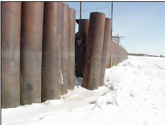
Pile wall of current concern at Bethel.
