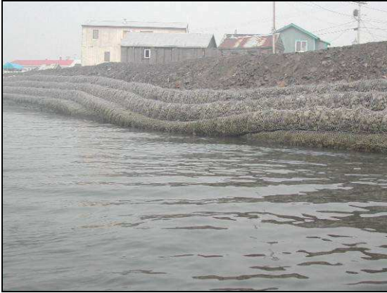
Sagging Gabion Wall
