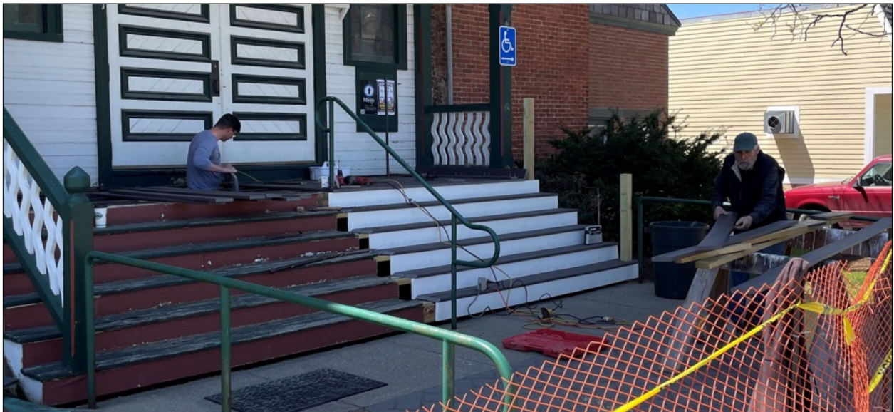
Zac Farnham-Haskell and Ted Lylis working on the porch and stairs replacement. Photo: Valerie Capels
