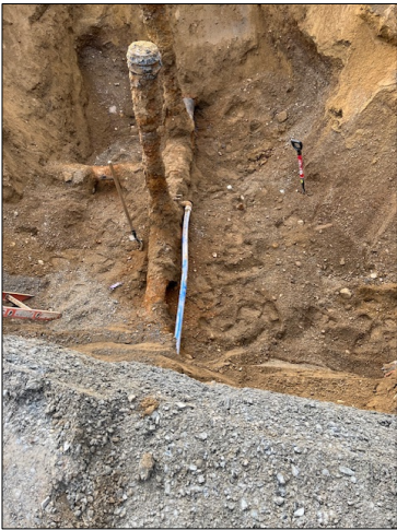
1905 Cast Iron Water Main
