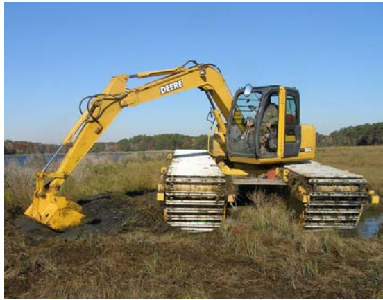
Amphibious excavator used to install ditch plugs / Donald Webster, MD DNR Wildlife & Heritage
