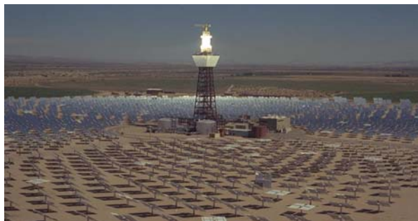
Solar Power Tower
