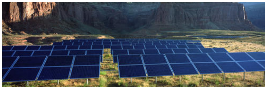
Solar Photovoltaic Power Plant
