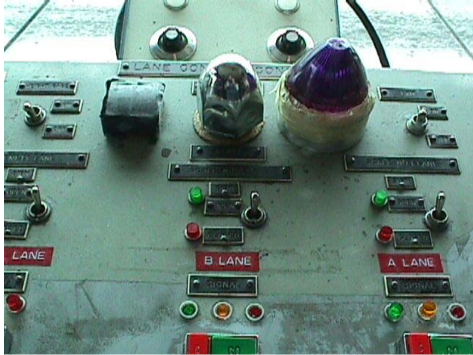
Figure 2.9. Control Panel at Castaic Weigh Station (California)
