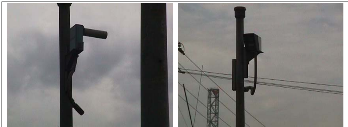
Figure 2.8. Detector System at Castaic Weigh Station (California)
