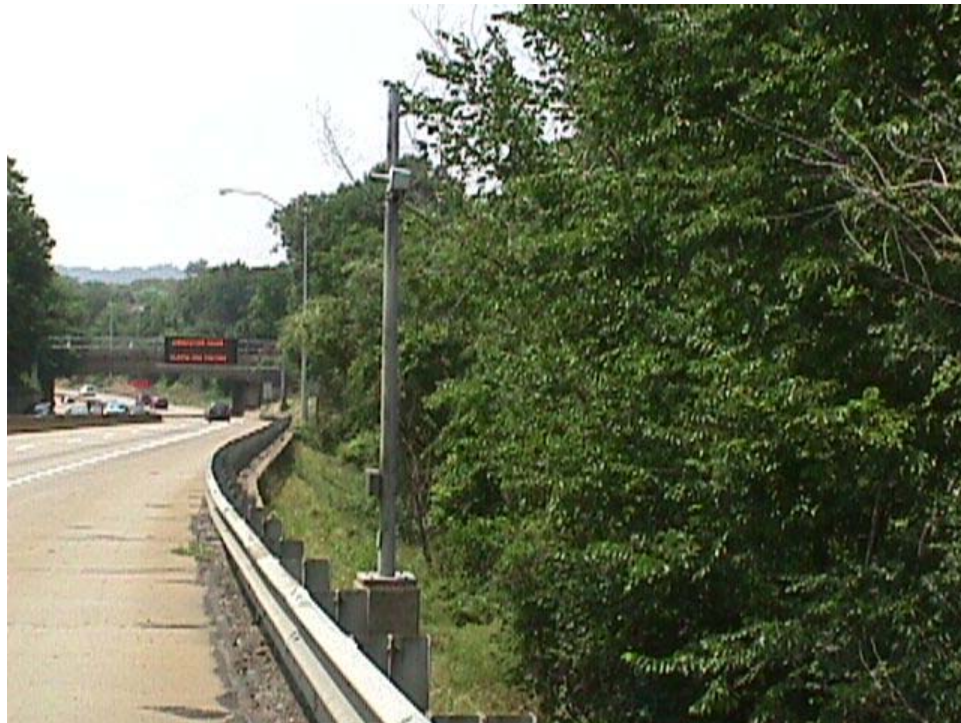
Figure 2.4. Upstream laser overheight detector on a standard pole
