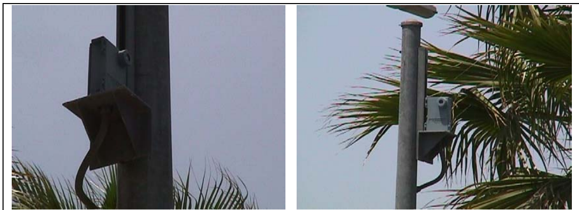
Figure 2.10. Detector System at Otay Mesa Weigh Station (California)
