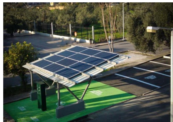
Figure 2. Experimental solar-based Electric Vehicle Charging Station (SEA Lab).
