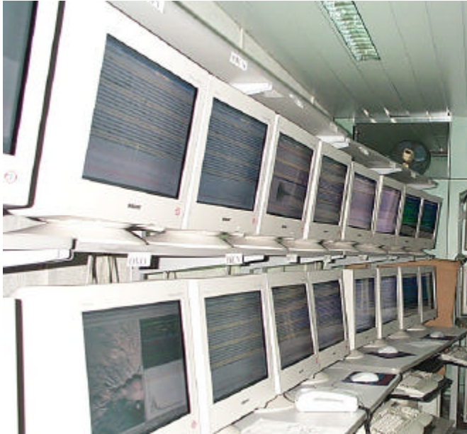
Fig. 4 – A view of the Osservatorio Vesuviano seismic monitoring system
