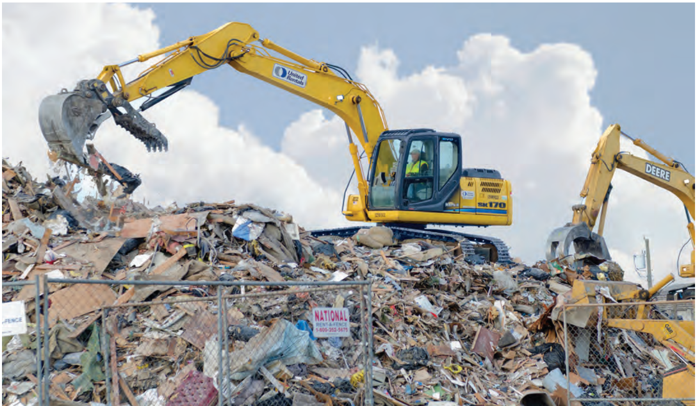
Hurricane Sandy debris in New Jersey
