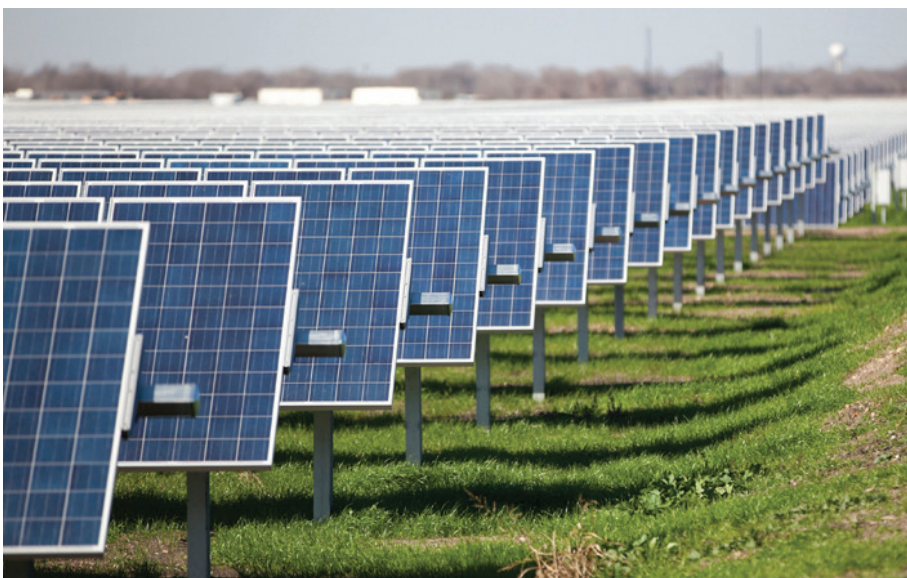
The 35 MW Webberville Solar Farm.
