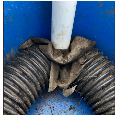
Figure 5. Filter/landscape fabric is placed in the void to prevent soil from entering the cut ends of the perforated pipe.
