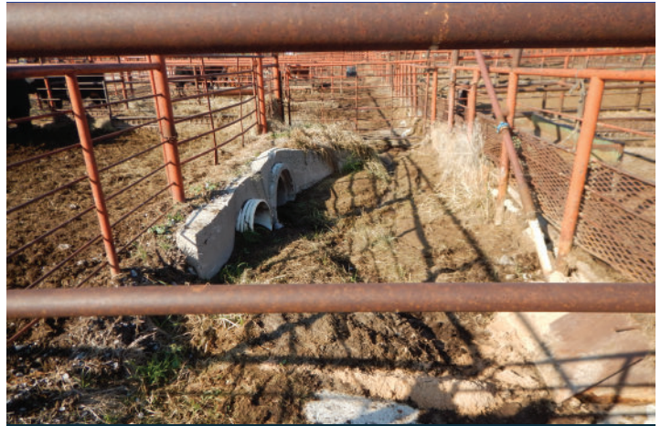
Photo 7: A drainage system of culverts and catchment basins directs all process wastewater to the facility's retention control structures.
