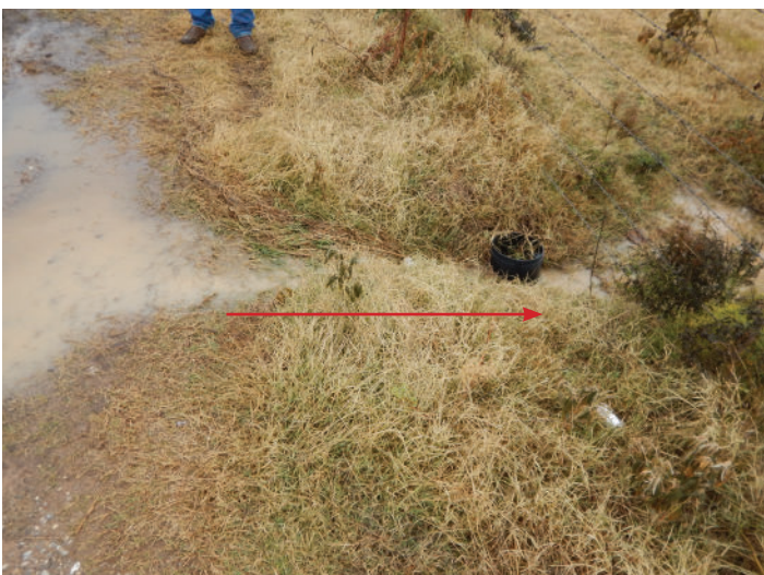
Photo 5: Process wastewater flowing off a manure and lot scraping storage pile due to incidental damage to the berm.
