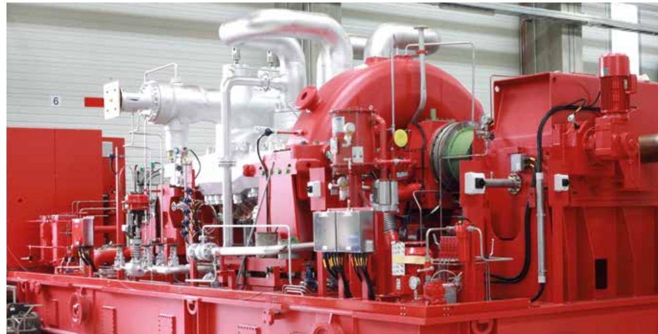
Biomass district heating plant, Västergötland / Sweden
