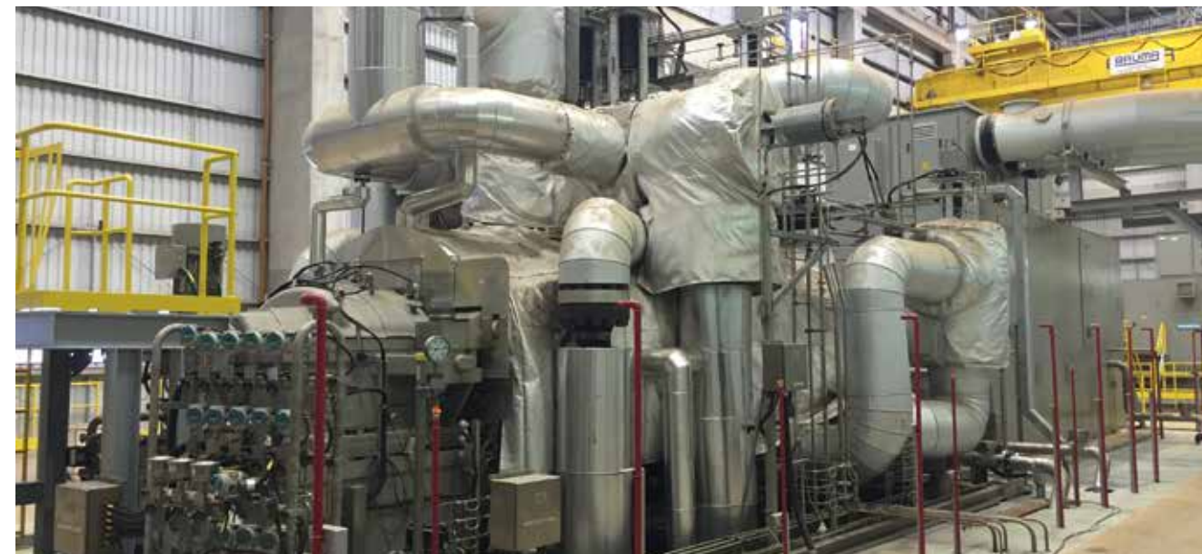
Steam turbine for the pulp plant Klabin, Brazil
