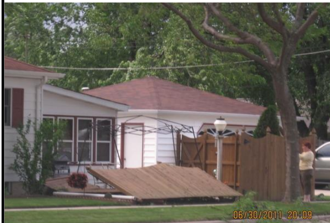
Kenosha – Fence Damage
