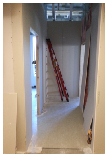
Requirement of a second access door to ATG 310 reduced the size of ATG 308 and extended the hallway.
