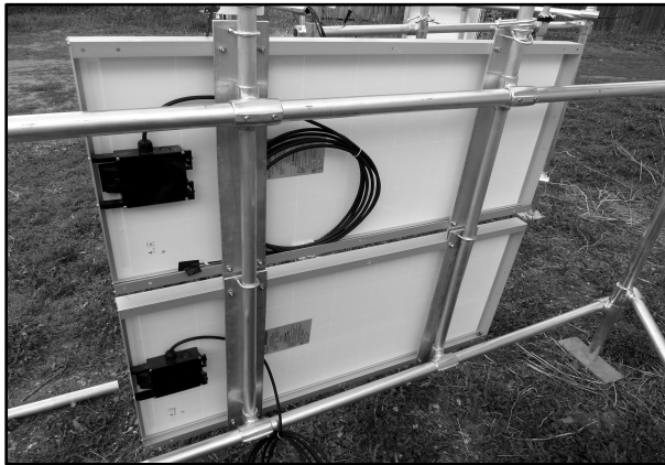
Figure 9. Dual 70 W solar panels mounted on tower cross arms. We have used Nu-Rails, U-bolts and aluminum plates to mount the panels, but many different configurations can easily be used for mounting.
