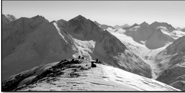
Figure 15. Alaska Rendezvous Guides crew completing site preparation for tower high on the shoulder of Mount Tiekle in the Chugach Range.
