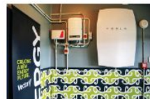
DISTRIBUTED ENERGY STORAGE
