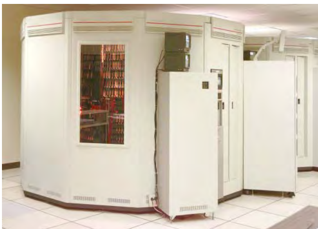
StorageTek 9310 tape silos
