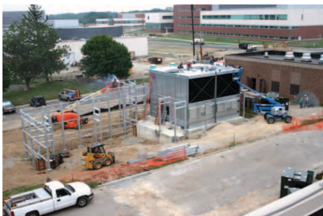
Pictured above, workers install two 600-ton cooling towers with pipe stanchions that will support the interconnecting feed and return pipes that will provide a balanced environment for the XE6 to operate efficiently
