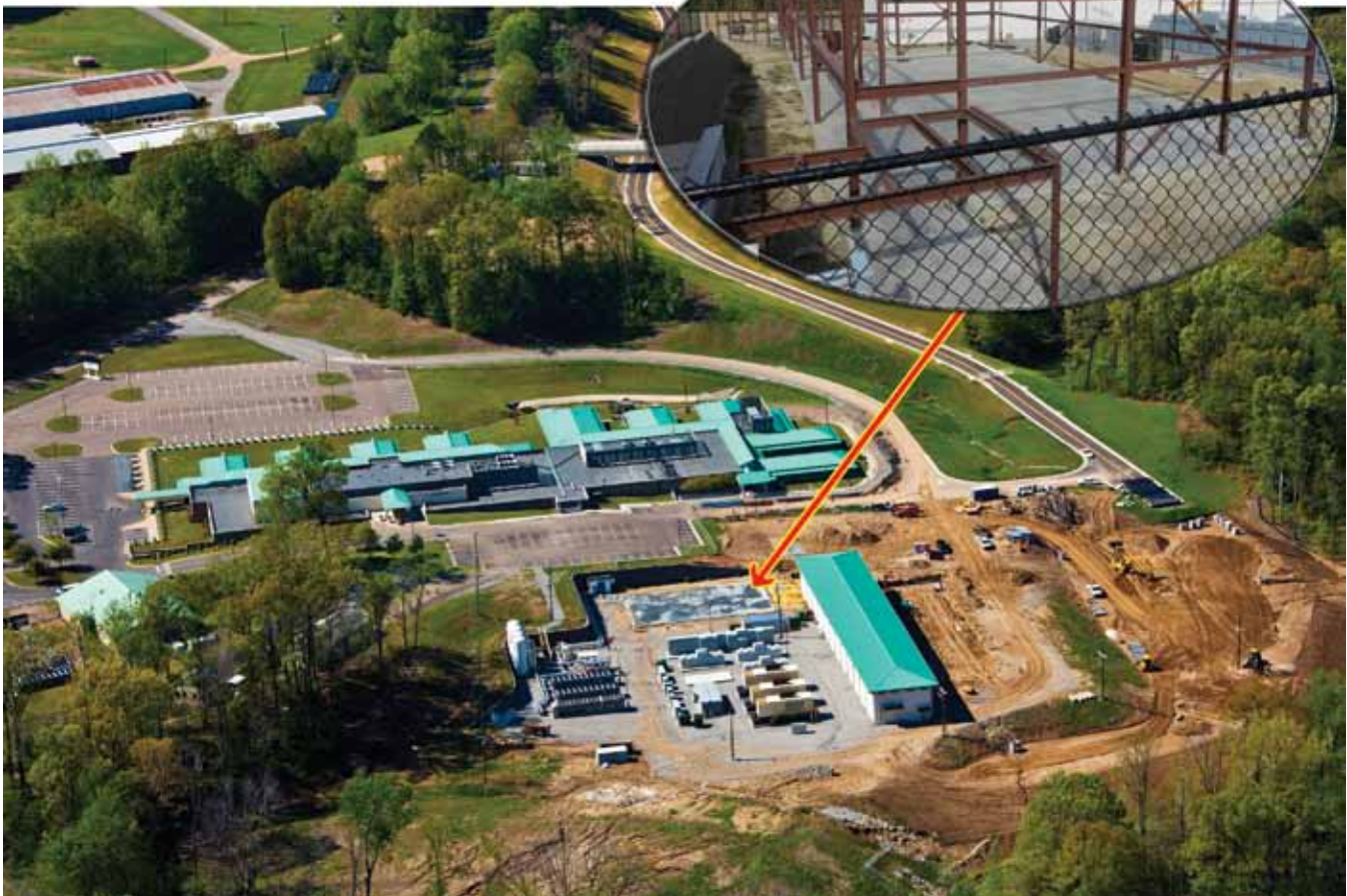
Aerial view of construction at ERDC Information Technology Laboratory earlier this year. Insert is more recent view showing office space and auditorium being built around supercomputer floor space.
