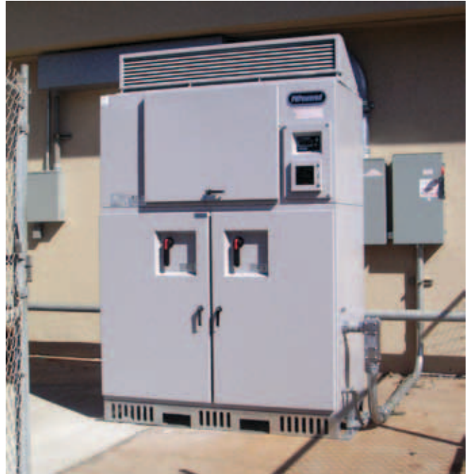
100 kW Inverter at the MHPCC Data Center
