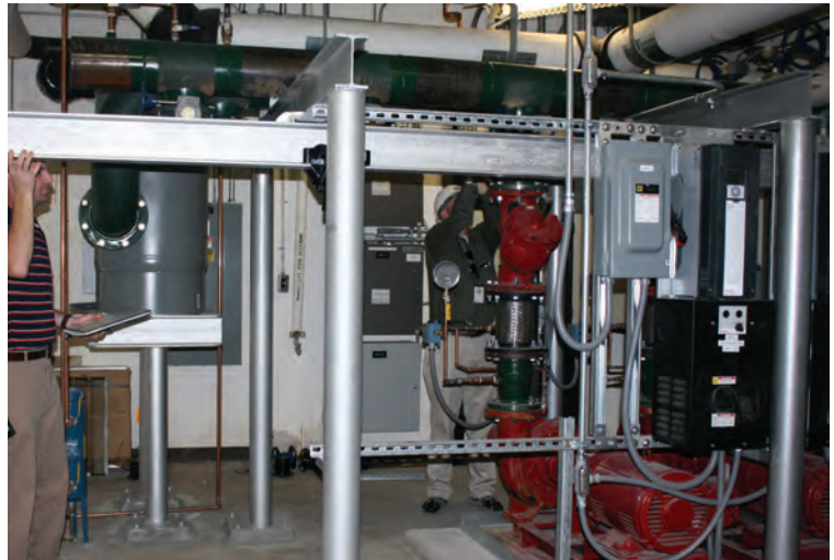
Facilities personnel oversee implementation of Center's secondary "cold" chilled water loop that will increase efficiency and flexibility
