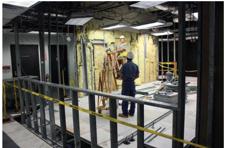
Remodeling of the computer operations room will improve system visibility and provide additional floor space
