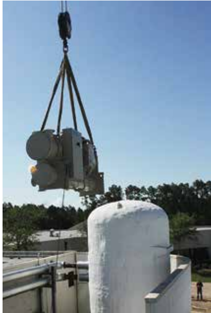
A new 300 ton magnetic chiller being lowered next to a 20,000 gallon cool water storage tank.
