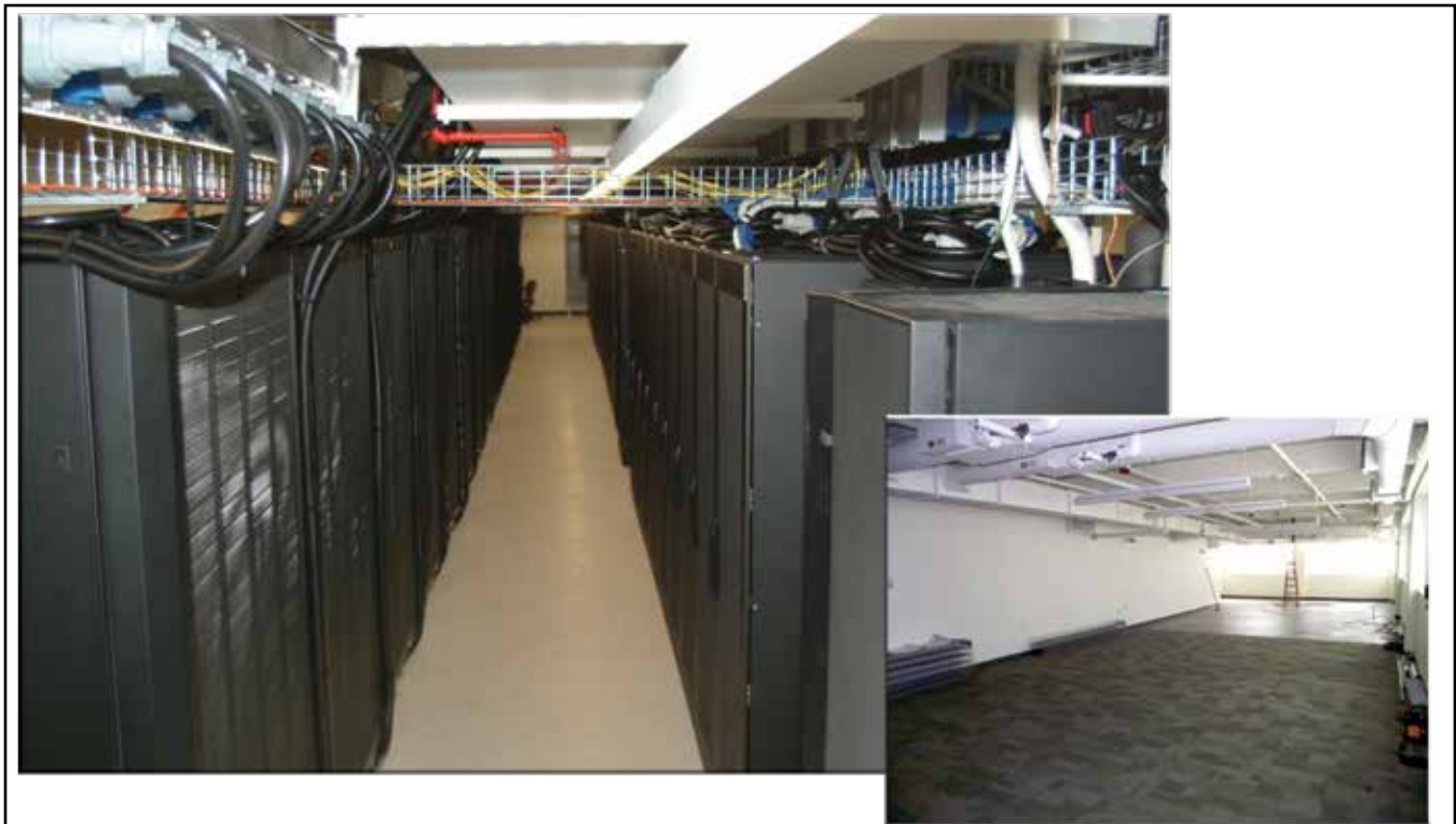
Blue Cell with Pershing system installed. (Inset) Blue Cell before conversion to computer room.
