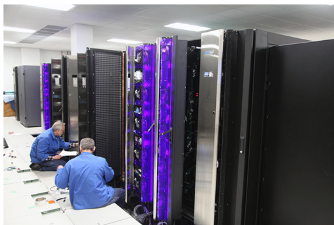
Workers install the miles of wire connections that network the thirty cabinets of the AFRL Cray XC30.
