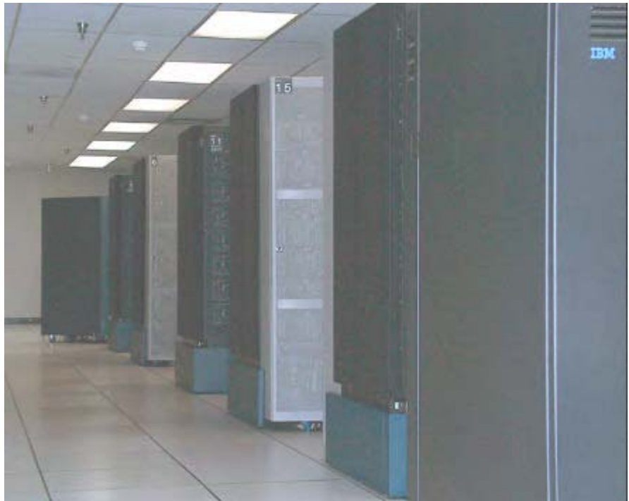
Looking down the aisle at many of the 24 cabinets which house Habu's 1.336 processors and massive storage capabilities.
