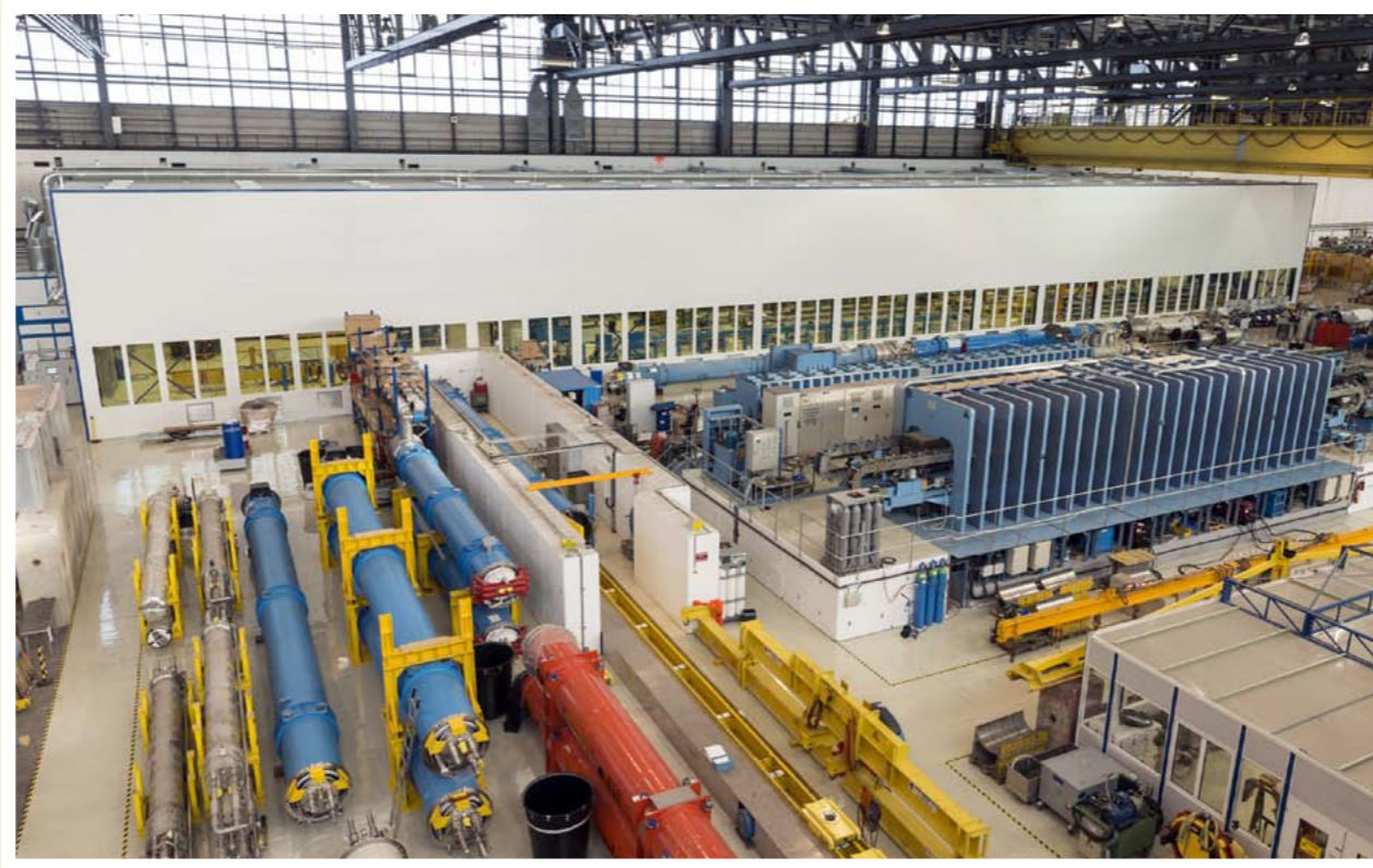
A view of the Large Magnet Facility in Building 180. To the left are spare cryomagnets, with the welding press on the right and the mock-up of a magnet string for training purposes just behind.
