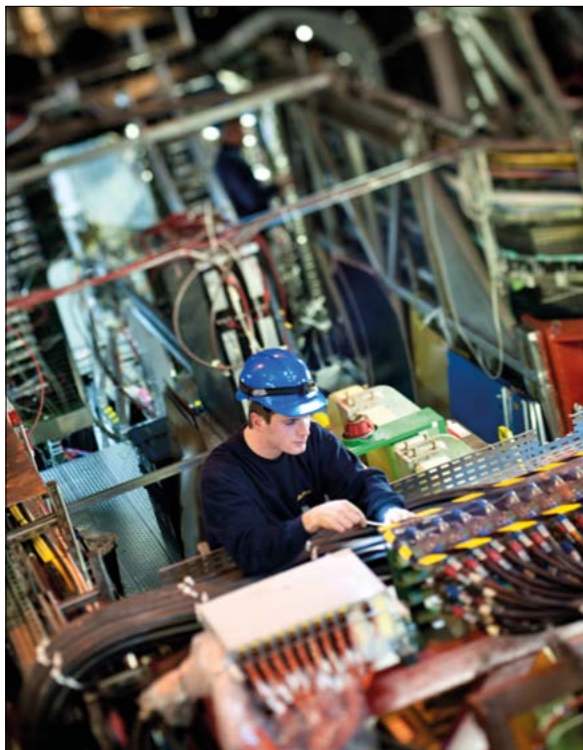
The consolidation of services, which includes air ducts, water ducts, high- and low-voltage power cables, optical fibres etc., will be one of the major activities during LS1. (Image credit: Antonio Saba/ALICE.)
