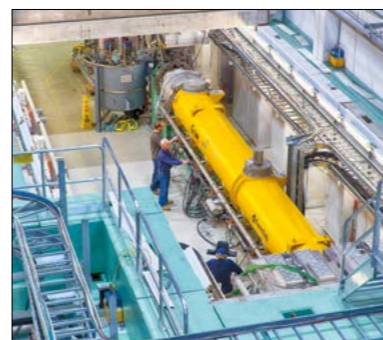
CM2 in its home at Fermilab's NML building, as part of the future Advanced Superconducting Test Accelerator. (Image credit: Fermilab.)
