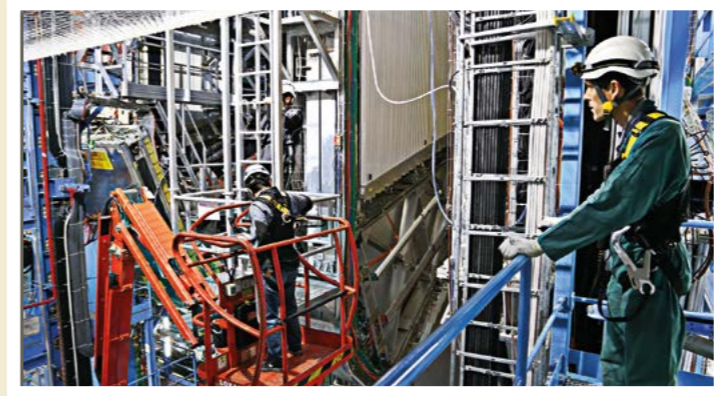
Above: Raphaël Vuillermet, the technical co-ordination team's engineer, supervises the separation of the muon spectrometer's big wheels from the cavern balcony. There are four moveable big wheels at each end of the ATLAS detector, each measuring 23 m in diameter. The wheels are separated to access the interior of the muon stations to change faulty chambers. (Image credit: Claudia Marcelloni.)
