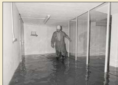
This swimming pool in the basement of the Main Building illustrates how the unusual volume of water far exceeded the capability of the drainage system.
