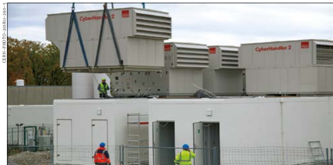
Under construction Modules being lowered into place for LHCb's new data centre.
