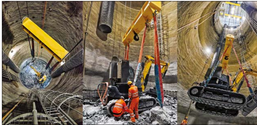
Digging for success The excavation of the two new shafts for the HL-LHC at points 1 and 5 of the accelerator has recently been completed.
