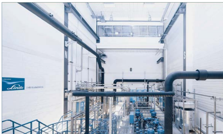
Example of a cryoplant, courtesy of Linde Kryotechnik AG.
