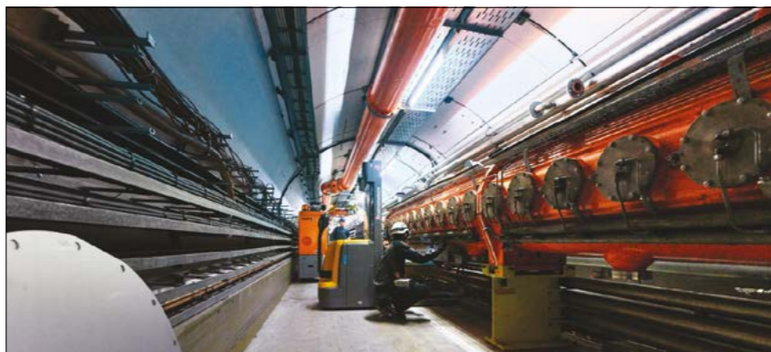
Workhorse Engineers in the SPS tunnel during the current long shutdown of CERN's accelerator complex.
