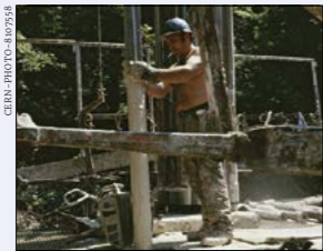
Drilling a borehole along the proposed line of the LEP tunnel in 1981 to reveal conditions likely to be encountered during excavation.
