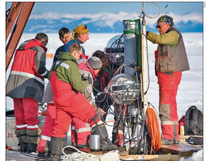
Ice breaker New clusters of optical modules being installed in the underwater Baikal-GVD Neutrino Telescope in April 2020.
