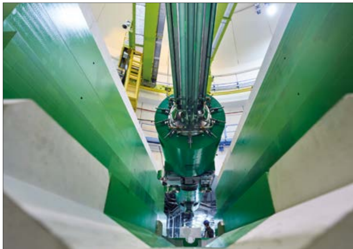
Structural integrity The new Super Proton Synchrotron internal beam dump being installed inside its shielding in October 2020.
