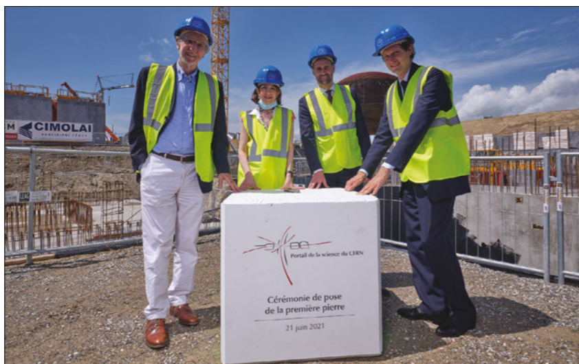
First stone (from left) Architect Renzo Piano, CERN Director-General Fabiola Gianotti, Geneva state councillor Antonio Hodgers and chairman of Stellantis and the FCA Foundation (the main donor) John Elkann with the symbolic foundation stone, adorned with the newly unveiled Science Gateway logo.
