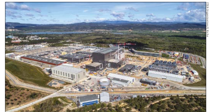
From above The 180-hectare ITER site in May 2021, with the 60 m-high assembly building seen in the centre.
