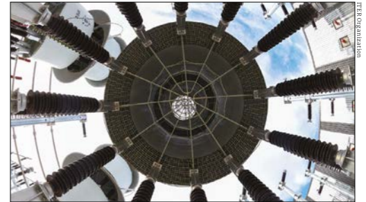
Input only Part of a power system to reduce harmonic distortions in the AC current that ITER draws from the grid.
