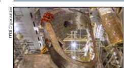
On the cover: An ITER vacuum-vessel sector docked in a sub-assembly tool on 6 April 2021. 34
