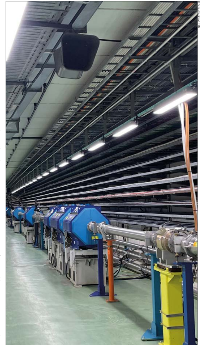
Linked up A section of the 300 m-long TT2 transfer line, which carries beams from the Proton Synchrotron to the majority of CERN’s facilities.
