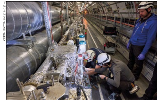
Crystal collimators Installation of new crystal collimators in the LHC tunnel at Point 7 in 2023.
