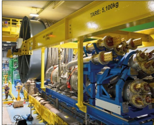
Cool technology The innovative cold-powering system for the High-Luminosity LHC was successfully installed in the inner-triplet-string test stand above ground in September.
