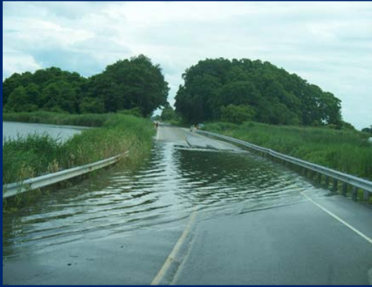
SR-9 near Port Penn floods during high tide and rain events, Middletown Transcript
