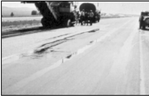
Figure A.6. Rutting
