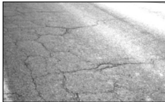
Figure A.7. Map cracking
