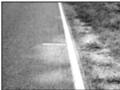
Figure A.5. Edge cracks
