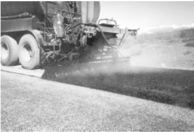
Figure 7.17. Emulsified asphalt distributor in action on the second coat of a double-layer AST
