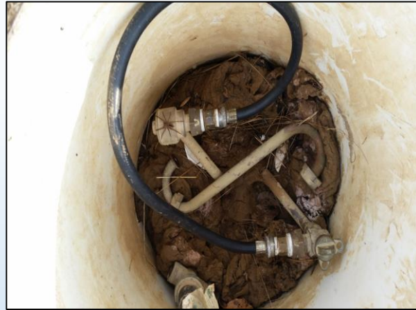
Hose used as Jumper Connection
