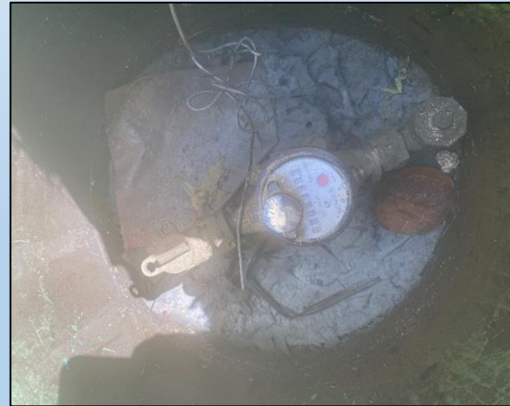
Meter register was removed and radio transmitter wire was cut
