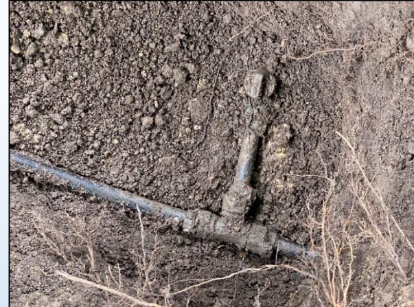
Un-Metered Connection – illegal by-pass with professional installation
